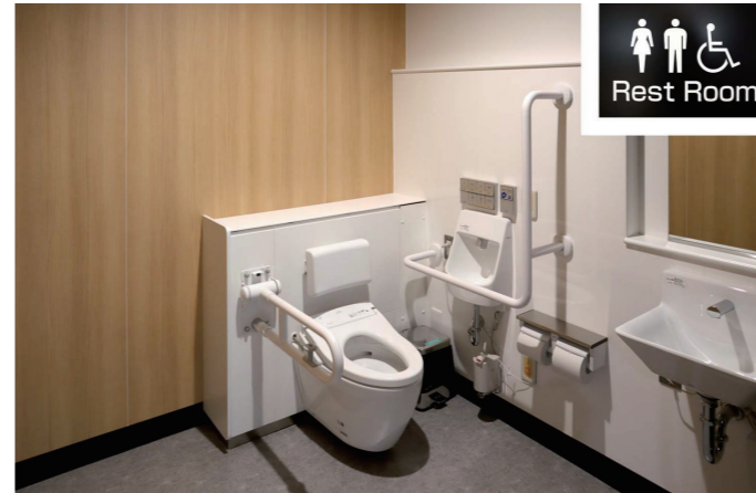
1F Rest Room①
